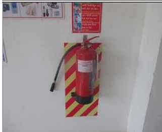
Photo of fire safety equipment Fire extinguisher.JPG
