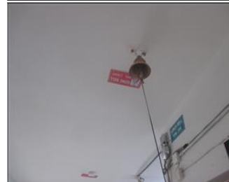
Photo of fire safety equipment Gong bell.JPG
