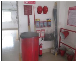
Photo of fire safety equipment Firefighting equipment.JPG
