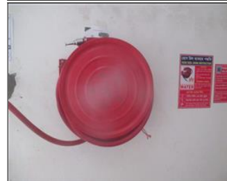
Photo of fire safety equipment Fire hose pipe.JPG
