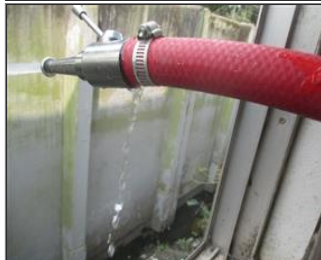
Photo of fire safety equipment Fire hose pipe demonstration.JPG
