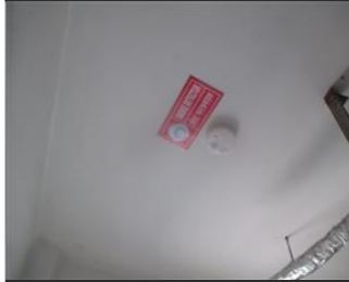
Photo of fire safety equipment Smoke detector.JPG
