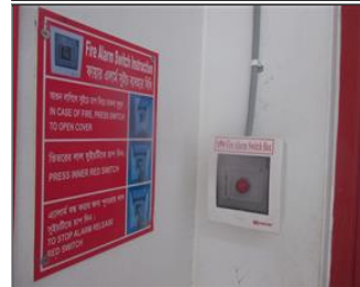
Photo of fire safety equipment Fire alarm switch.JPG
