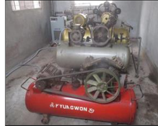
Photo of non-conformity Compressor found without safety barrier.JPG
