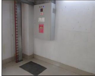
Photo of the inside of the main production hall Power Distribution board.JPG
