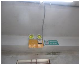
Photo of fire safety equipment Emergency light.JPG
